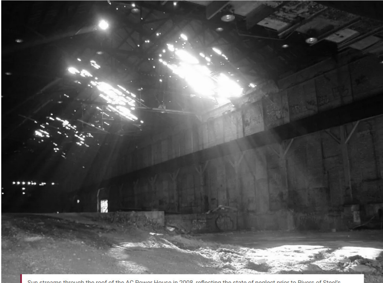
Sun streams through the roof of the AC Power House in 2008, reflecting the state of neglect prior to Rivers of Steel's stewardship. Photo by Ron Baraff.
